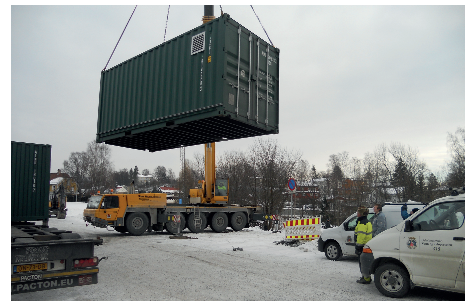
Figure 3: Installation of the local high-rate filtration unit at Hoffselva site in February 2015.
